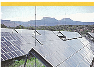
Sunica battery features: installed on Mt. Edwards (top photo) in the container under the solar panels, the pocket-plate technology features a special spill-proof vent and an extra electrolyte reserve that ensures almost supervision-free operation and a long interval between topping-up. Their expected service life-time can reach 20 years, and there's no risk of lead-acid's “sudden death”.
