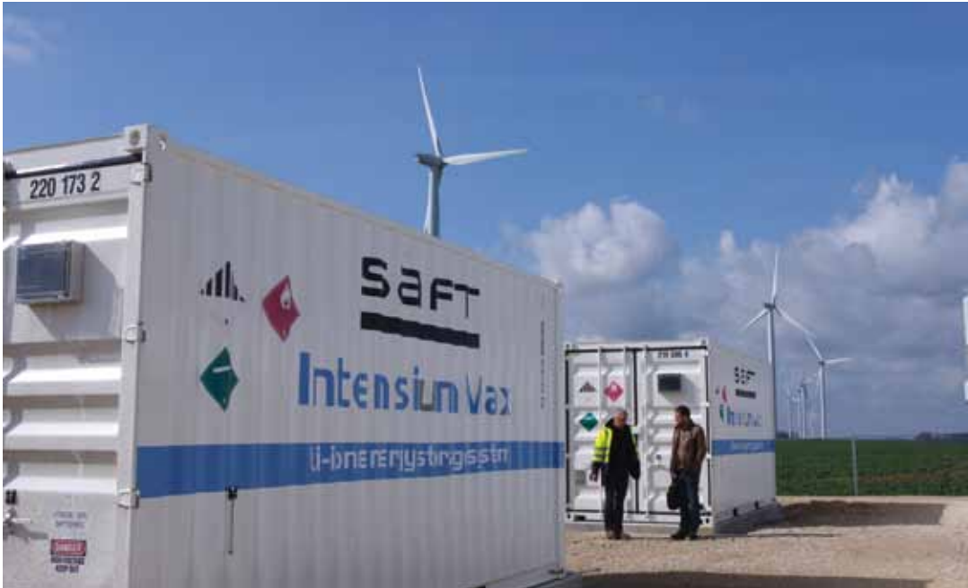
Venteea, the largest battery system ever to be installed in mainland France.
