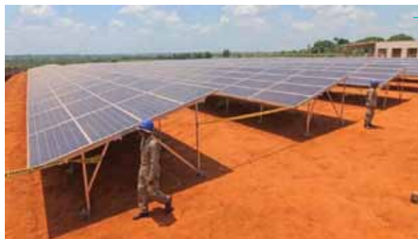
The hybrid power plant will coordinate PV and diesel generation to maximise the use of clean solar power to meet around half the energy demand in Pando's capital city Cobija and nearby towns.
