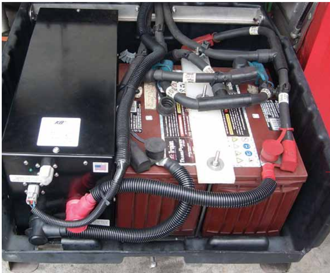
Saft Supercapacitor starting module built by KBI and installed in place of 2 batteries on New Flyer transit bus.
