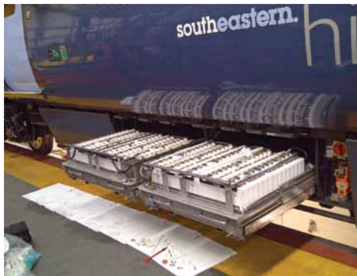
Refurbishing on-board batteries ensures their performance
