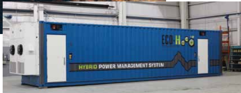
ECO-H partners a lithium-ion battery system with a diesel generator
